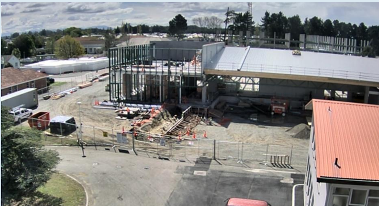
Below: View of Back of House at Burwood with half the roof now on.
