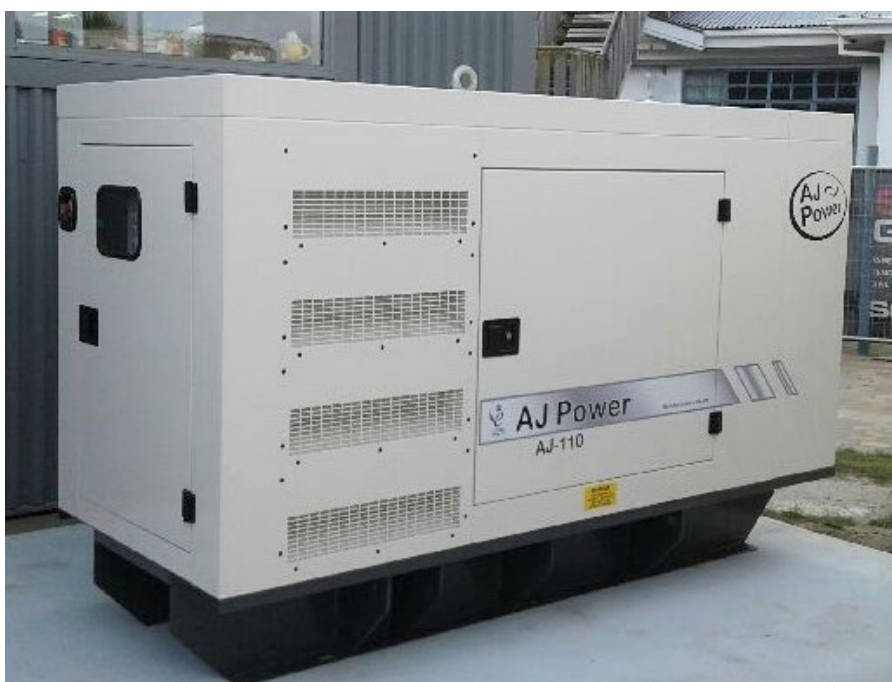
The new diesel-powered generator at Rangiora Health Hub
