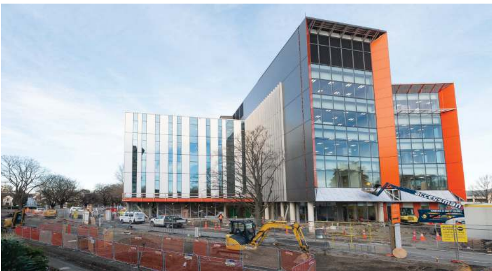
Standing at a gateway to the central city and the Health Precinct, the Outpatients building is a distinctive presence. The orange "eyebrow" features around the main windows are unmistakable and will help people find the new building.
