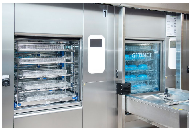
Some of the new equipment that sterilises medical devices
